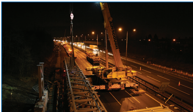
Construction team installing a gantry at night to avoid public disruption on the Birmingham Box Managed Motorways project.
